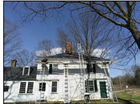
Because construction work is considered essential under the stay-at-home order, Hinsdale House got its new roof.
